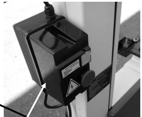
Switch in operation position
